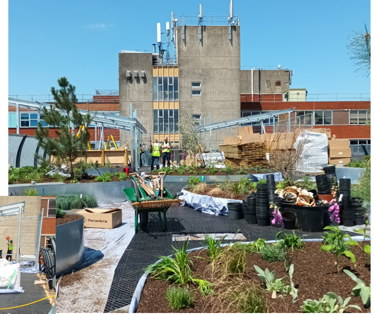
The project was constructed in Spring and early Summer 2023. Working in a live hospital environment with multiple crane lifts, road closures and 24hr access for staff required careful coordination and programming.
